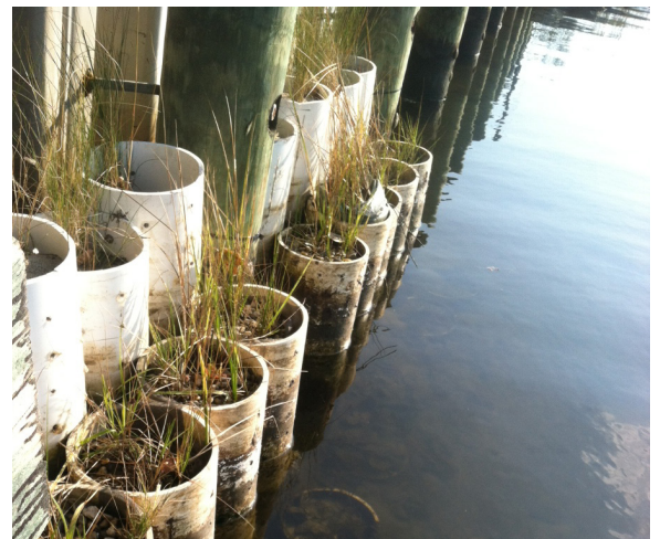
The completed installation of a green bulkhead in Ocean City. Grasses are planted in the top of these PVC pipes to provide additional habitat for fish and other aquatic species. Photo by Roman Jesien.
