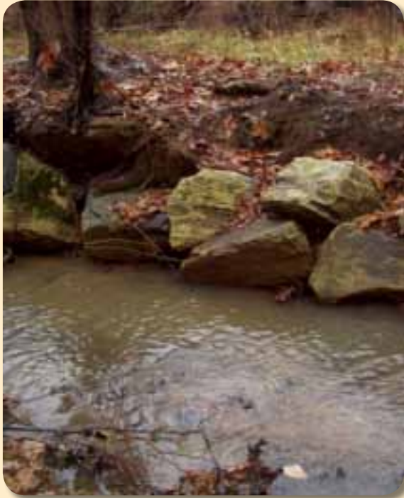
Stream restoration site with artificial stream bank installed to reduce further erosion.
