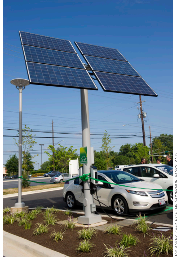
Tracking solar array to charge electric cars.
