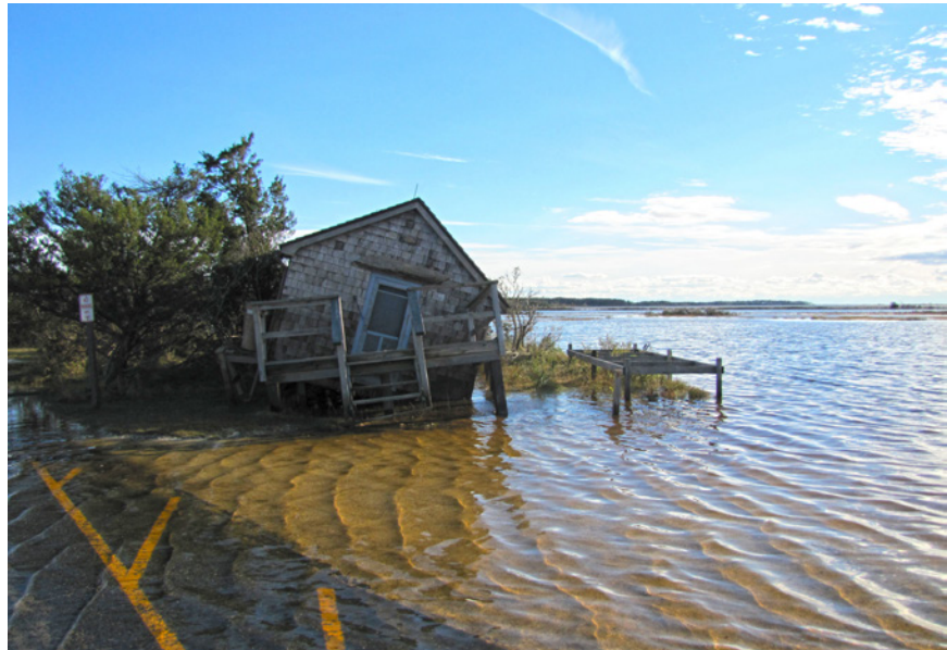
Assateague Historic National Seashore subject to considerable flooding, erosion, and infrastructure damage following Hurricane Sandy in 2012.
