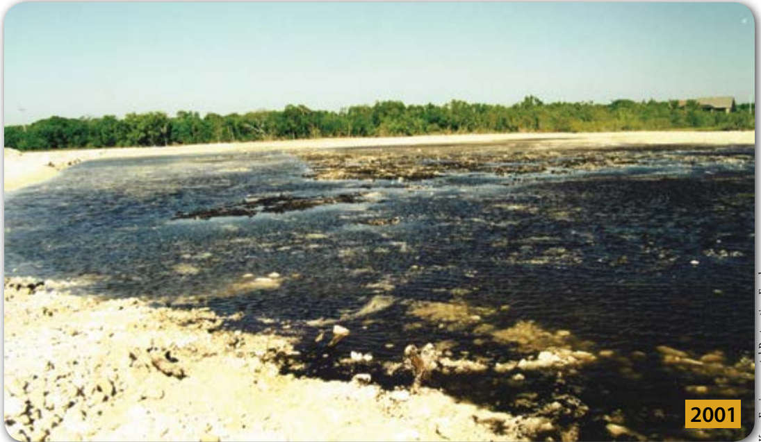
Carysfort Yacht Basin (2001) immediately after scrape down of fill material to natural grade.
