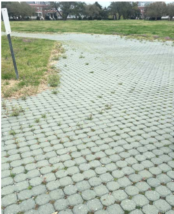
Pervious pavers in Fort Monroe National Monument (Photo credit: Todd Lookingbill, University of Richmond).
