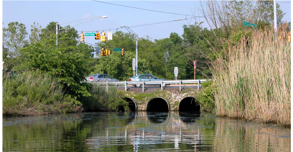
The beginning of a buried stream under Maryland State Road 322. These streams are redirected into pipes below the pavement.
