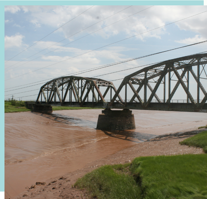
Erosion, flooding, and sea-level rise degrade and damage infrastructure. Future development should be built strategically with resilient communities and infrastructure in mind.
